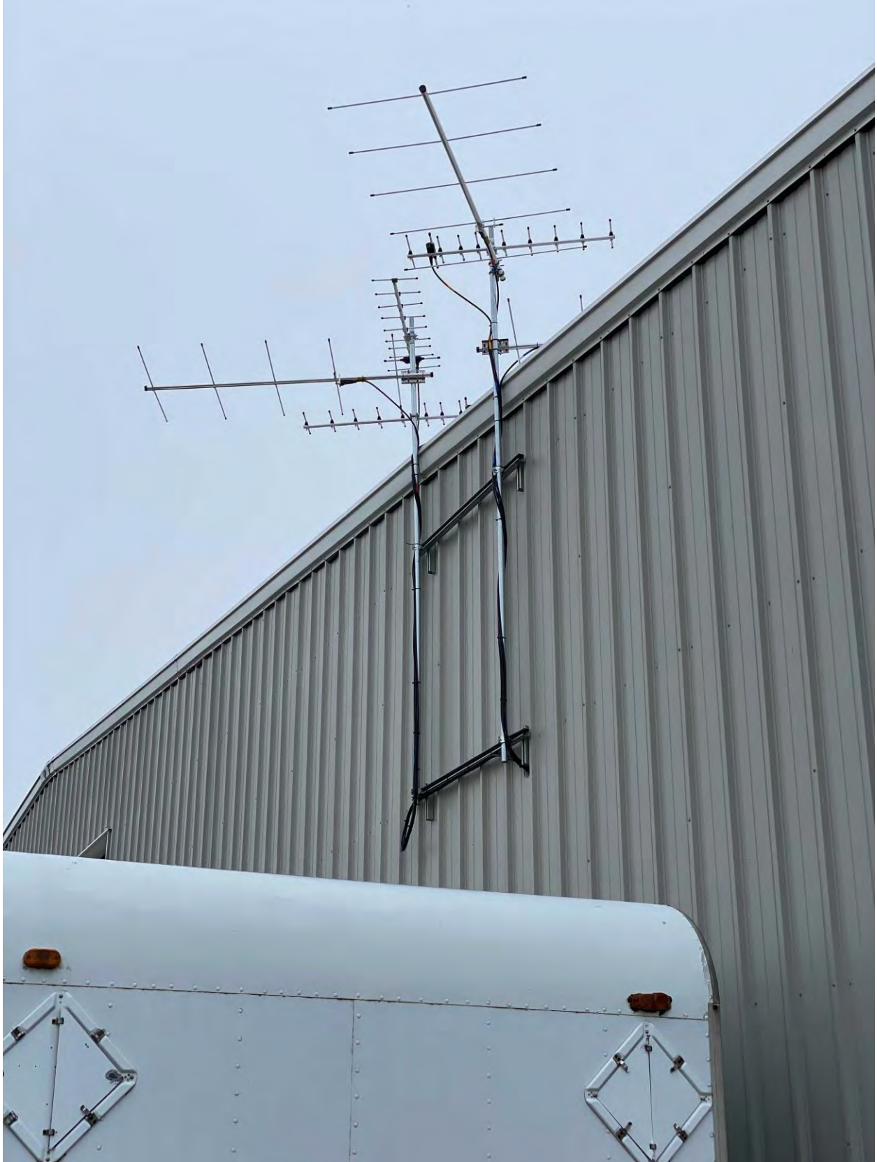
Motus station mounted on the side of a building with strut channels in California. Photo: Patrick Lorch
