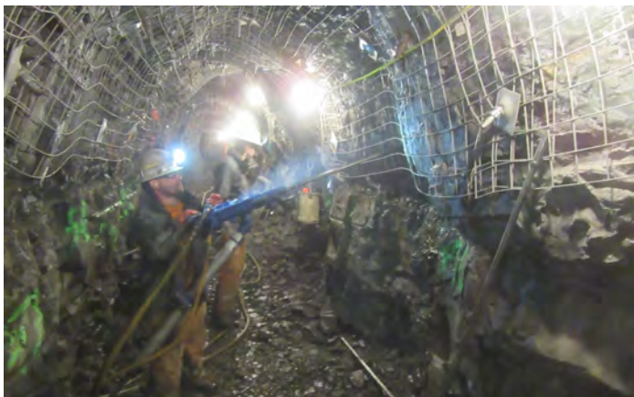
Refurbishing the existing rock support elements at the Peace Canyon left adit – a passage located in the dam abutment.
